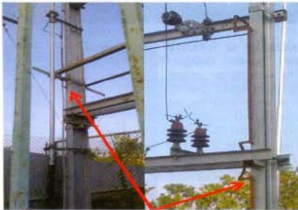
Earth conductor of Surge Arrester insulated from the structure
